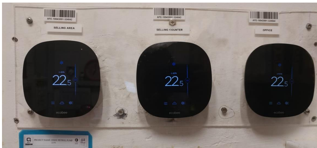
Fig.6. Automatic thermostats installed in ENOC 1079
